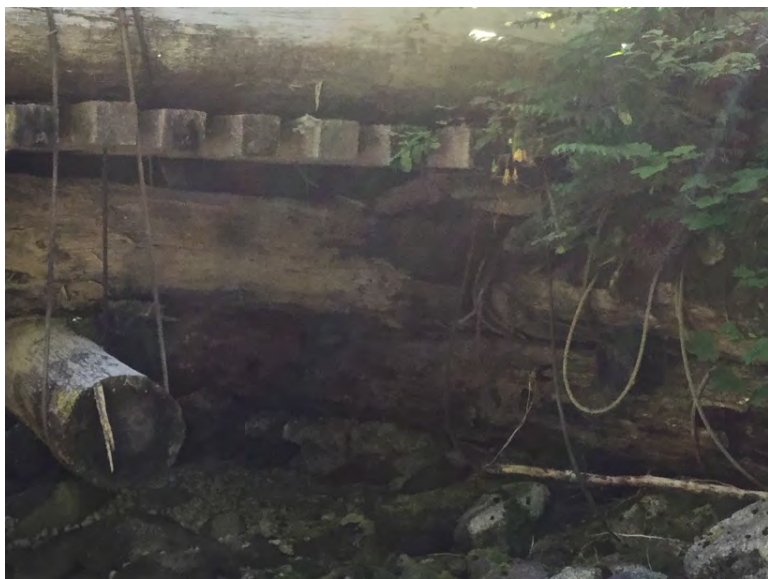
Downstream log stringer condition at left bank
